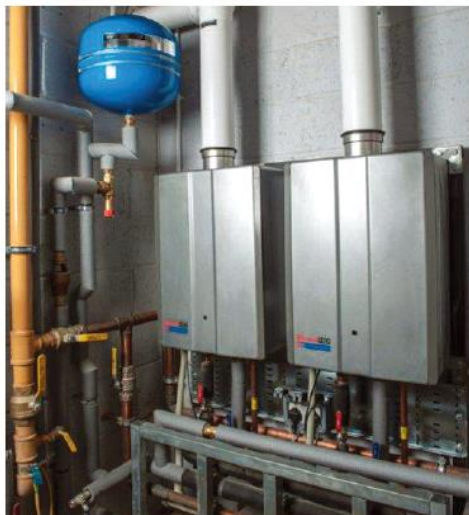
Figure 6: A pair of continuous flow water heaters installed to produce in excess of 1,400 litres per hour of hot water at 60°C (Source: Rinnai UK)
